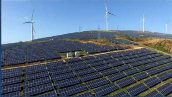
Fig. 1 Renewable Generation Plant
