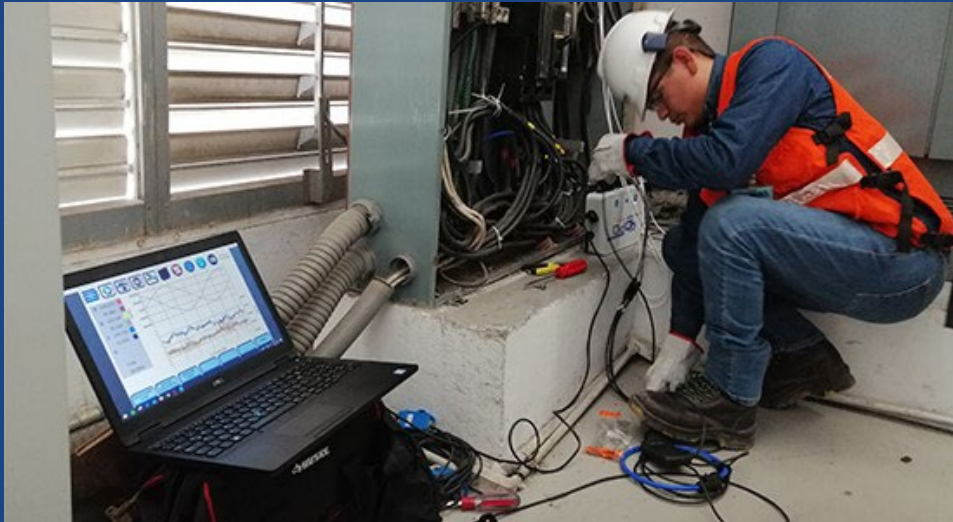
Fig. 1 Meter installation in distribution board.
