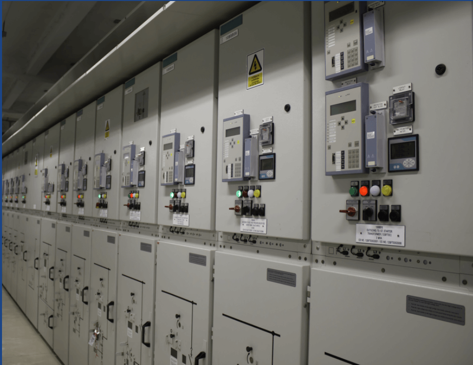
Fig 1 Metal clad switchgear.
