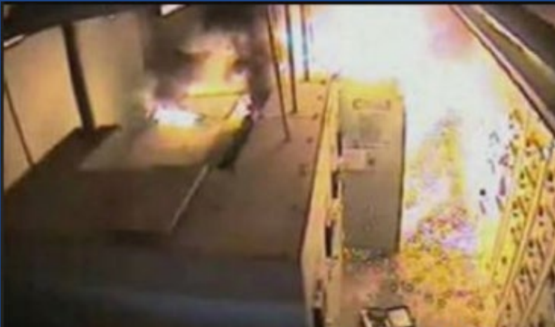
Fig. 1 Arc flash fault inside Metal-Clad switchgear.
